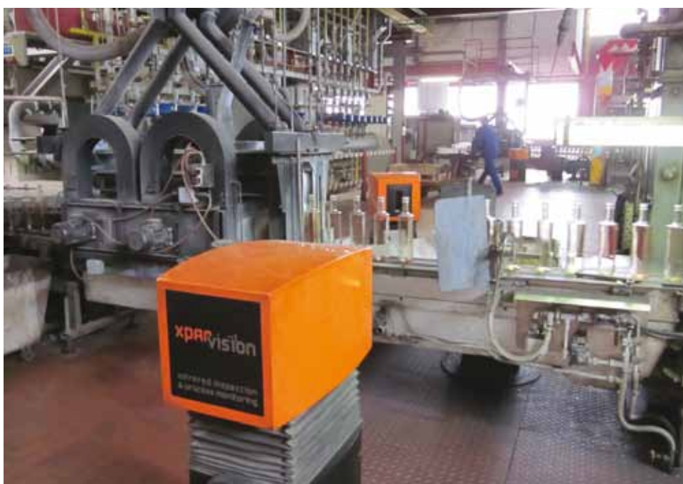
XPAR Vision infrared camera system installed at a Wiegand Glas plant.
